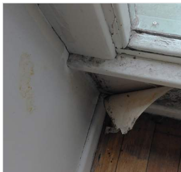
Actual photos of unsafe rooming house conditions.
